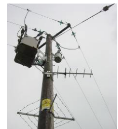
Distribution pole with radio-controlled switch.
